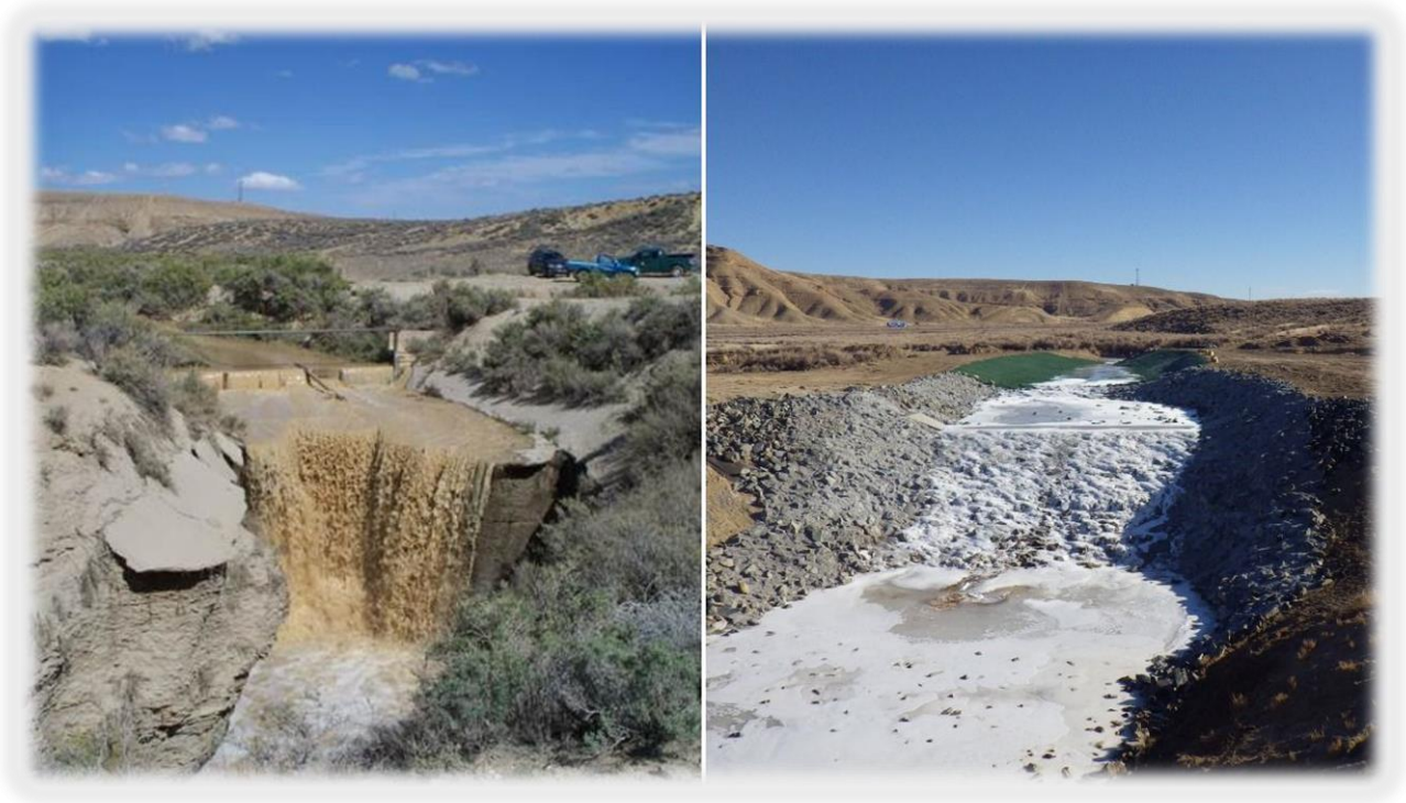
Left picture - Existing Drop Structure before construction of new channel and drop structure. Right picture - New drop structure upstream of existing Drop Structure
